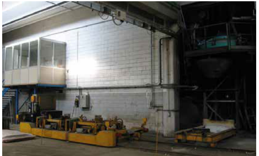
TROLLEY-BUCKET ON THE GROUND
